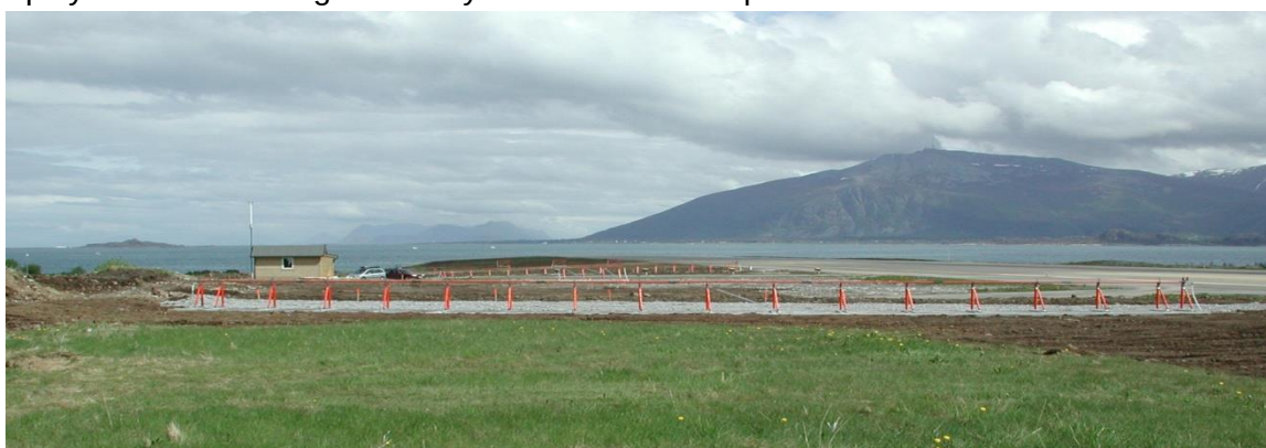
Endfire system glide slope installed at Vigra, Norge.
